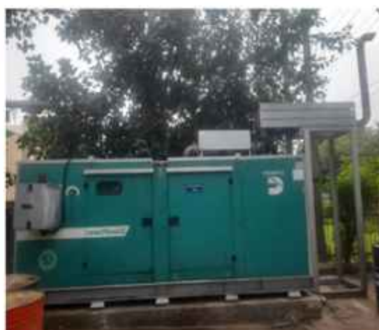
DG Set with retro-fitted ECD
