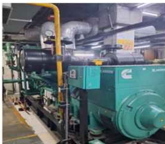
Dual Fuel System in DG Set
