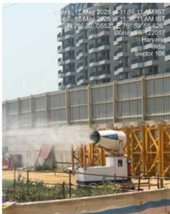
Anti-smog gun installed at project site
